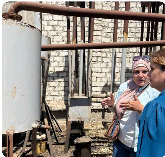
Dr. Maha El Attar walks Ms. Khalifeh through Carbonera's pyrolysis unit, Damanhour
